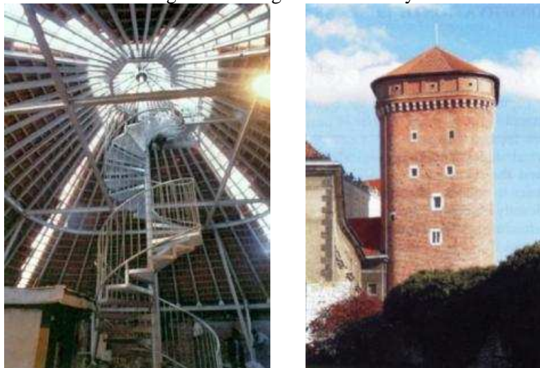
Fig. 7. The horizontal bracings in the steel reconstruction of the Lubranka tower roof on the Wawel (left) and a view of the object after completion of maintenance works (right) photo by P. Stępień [10]
