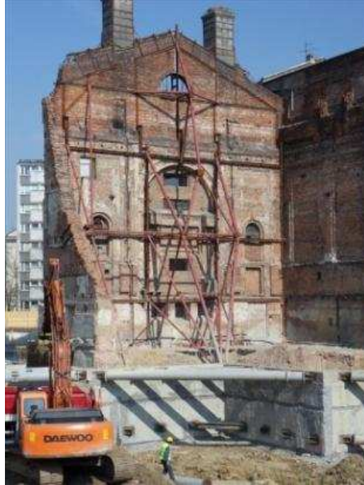
Fig. 2. Renovation bracing angle strut-cantilever type of historic front wall with a height of 28.0 m (designer - Cz. Hodurek) [3]
